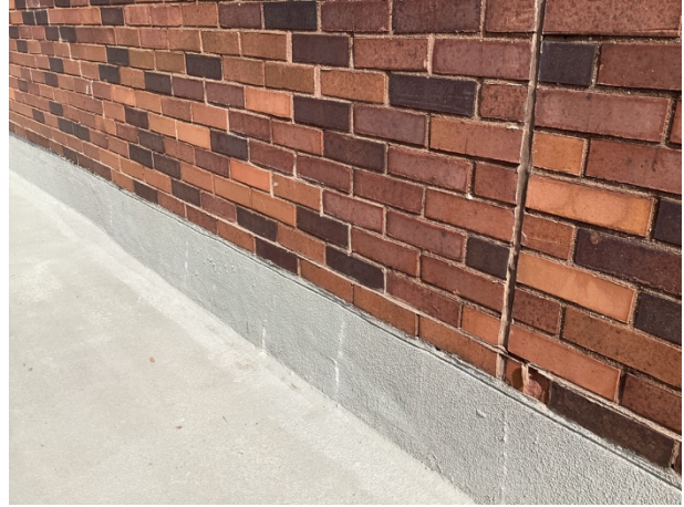
Spall at north wall
