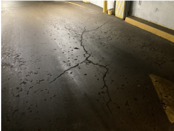
Concrete cracks and spall
