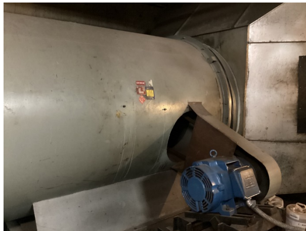
Exhaust fan for kitchens
