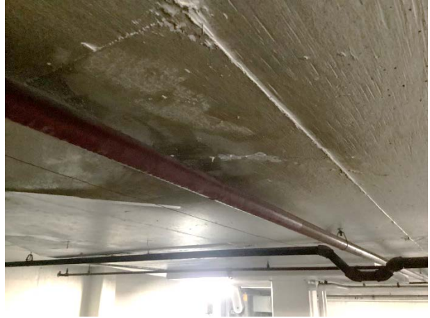
Evidence of past water infiltration beneath vaulted plaza
