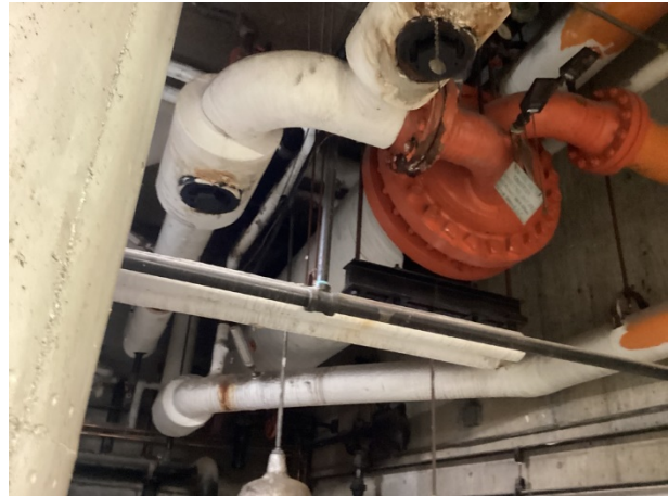
Mall heat exchanger
