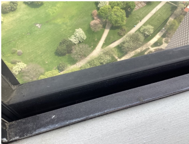
Deterioration of weather strip at operable window
