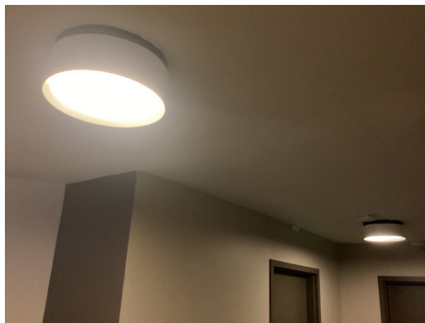
Fixtures at hallway
