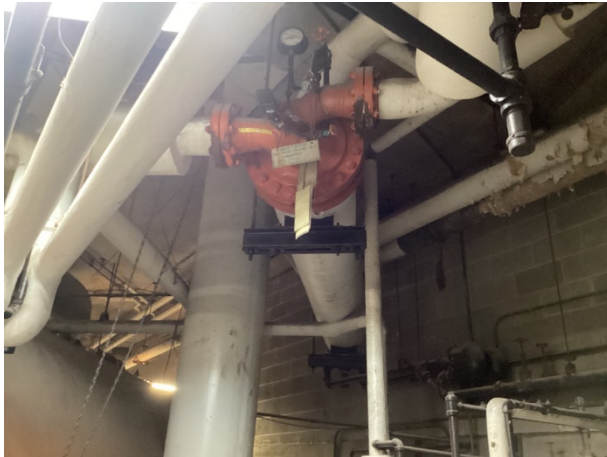
Fin tube heat exchanger
