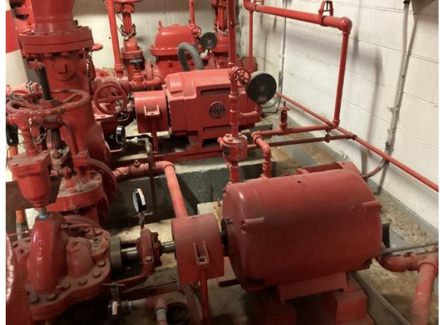
Fire suppression pumps
