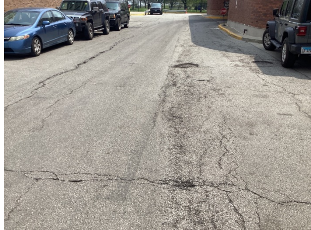
North asphalt pavement deterioration
