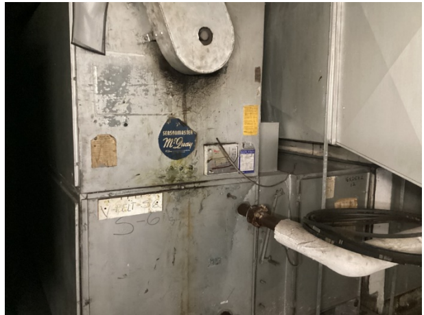
Mall air handling unit
