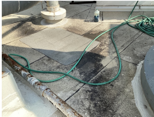
Main roof at repairs and lack of drainage
