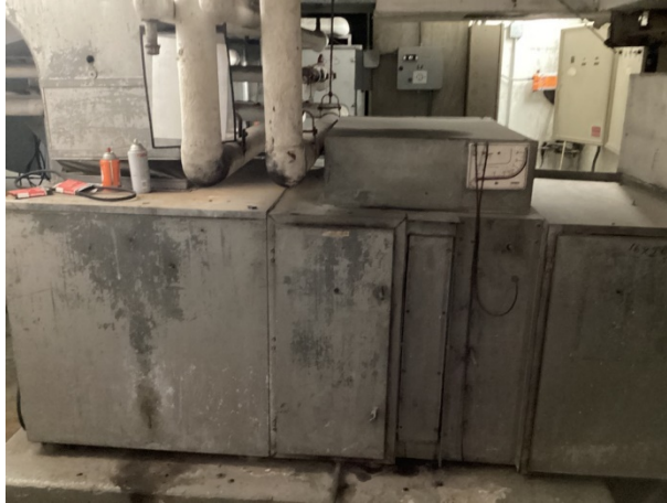
Party room air handling unit
