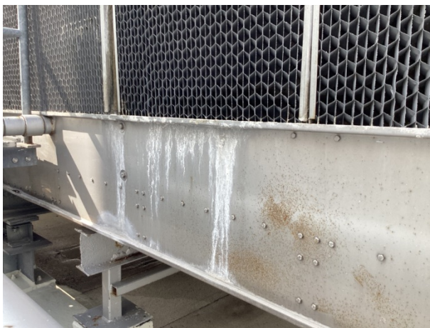
Cooling tower at leakage
