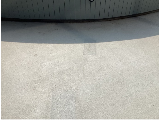
Cracks at 2nd floor coating
