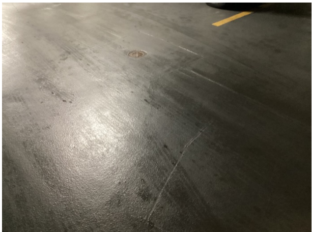
Concrete repairs beneath traffic coating
