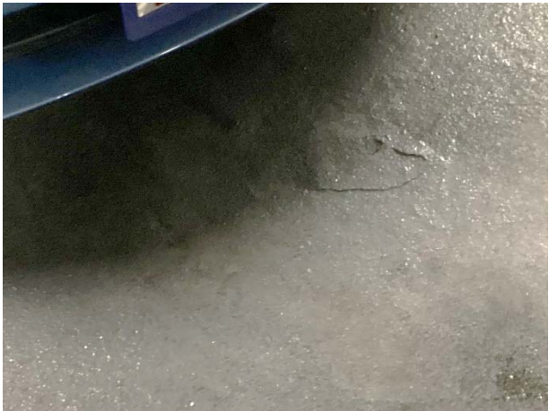
Traffic coating damage at valet
