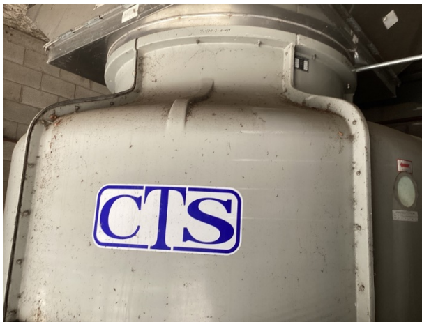
Commercial cooling tower
