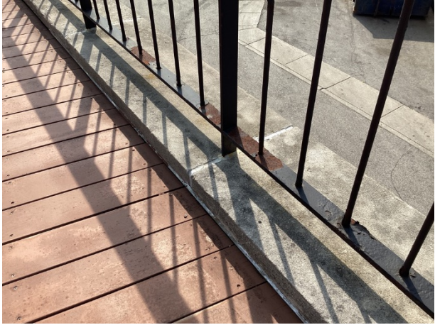
Corrosion at railing
