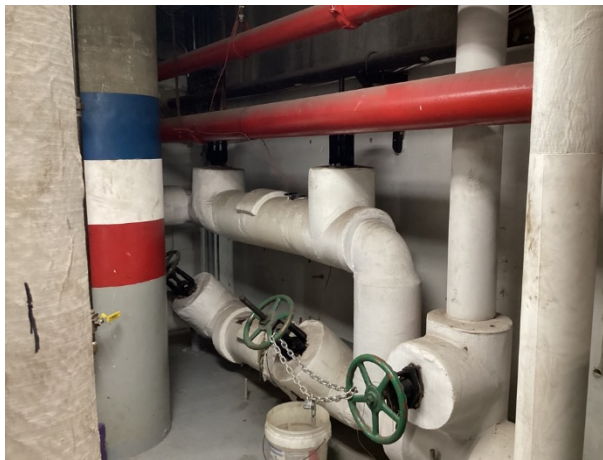
Main water connection large diameter valves
