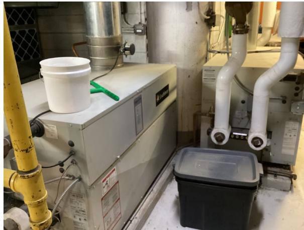
Low zone domestic water boilers
