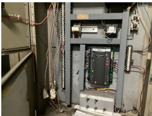
Building automation system panel
