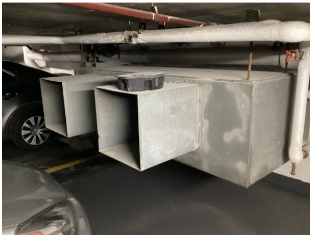
Garage air handler
