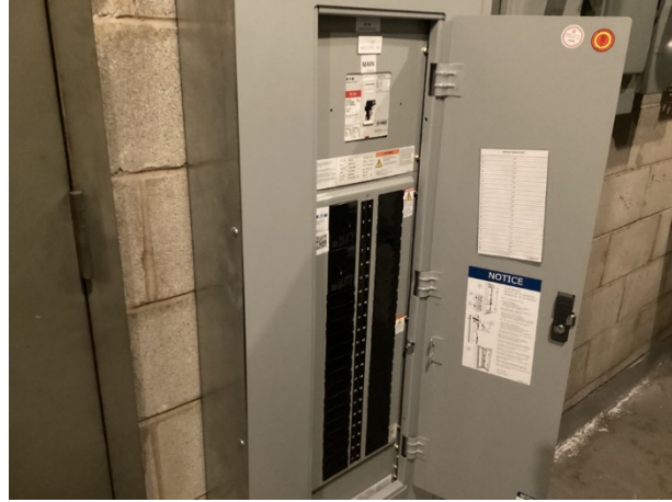
New circuit protection panel for charging stations
