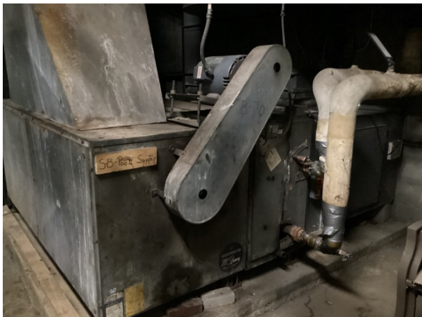
Pool air handling unit
