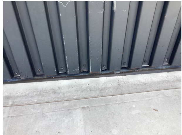
Siding corrosion at base
