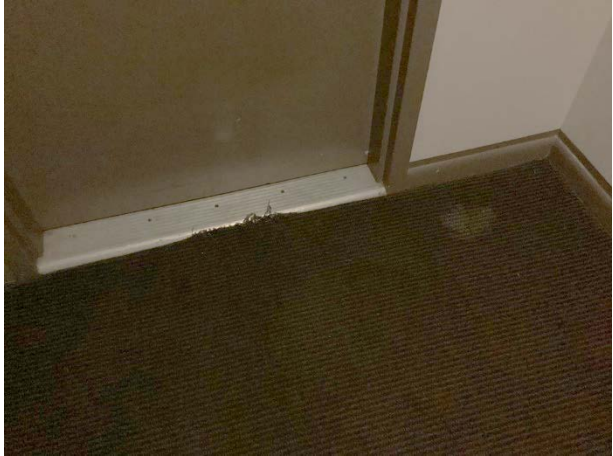
Carpet deterioration at edge
