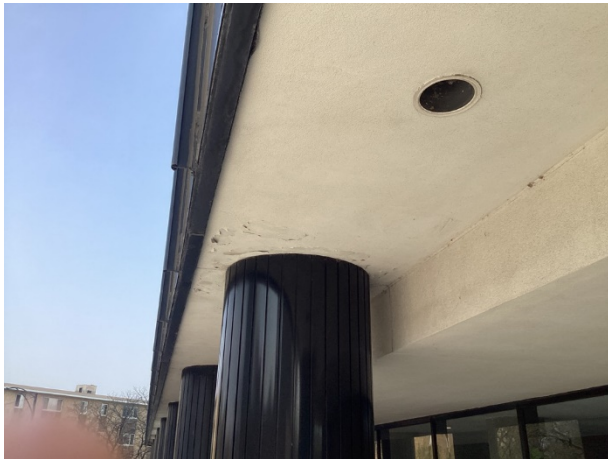
Soffit paint finish deterioration
