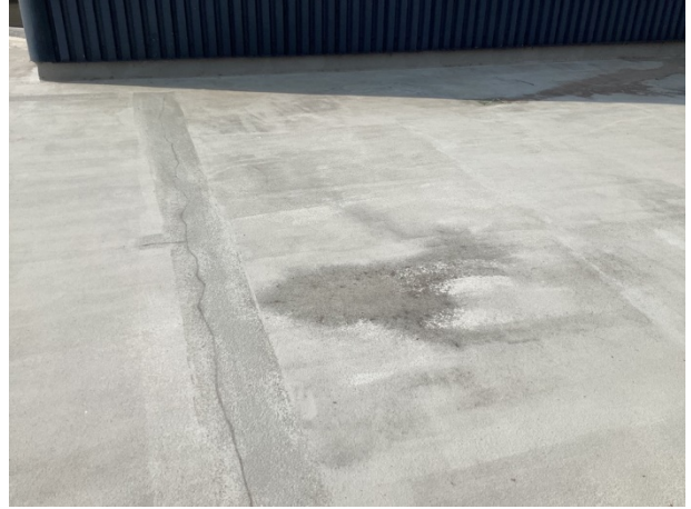
Lack of drainage at 2nd floor roof
