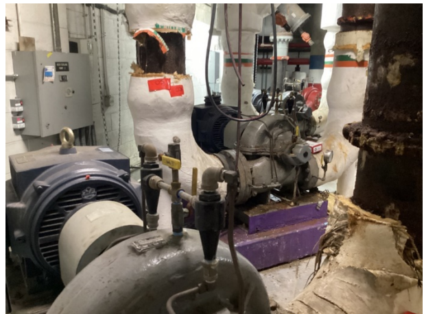
Fan coil loop pumps
