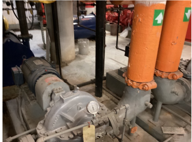
Commercial heating pumps
