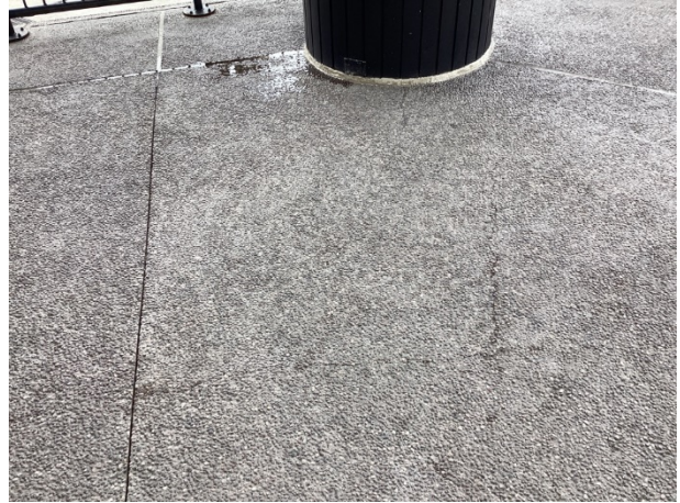
Cracks at plaza
