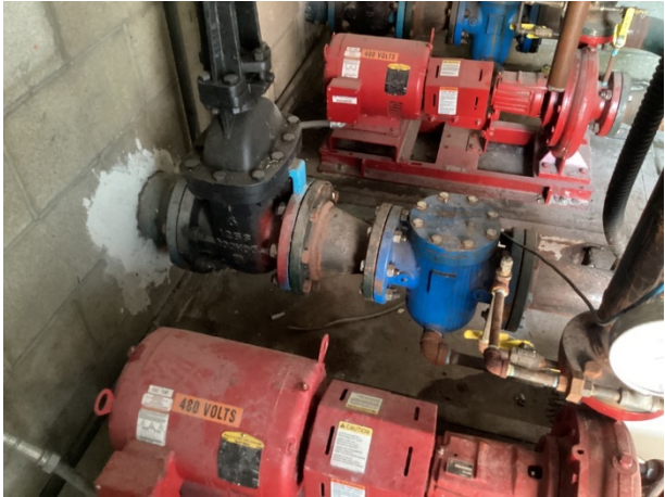
Commercial cooling tower pumps
