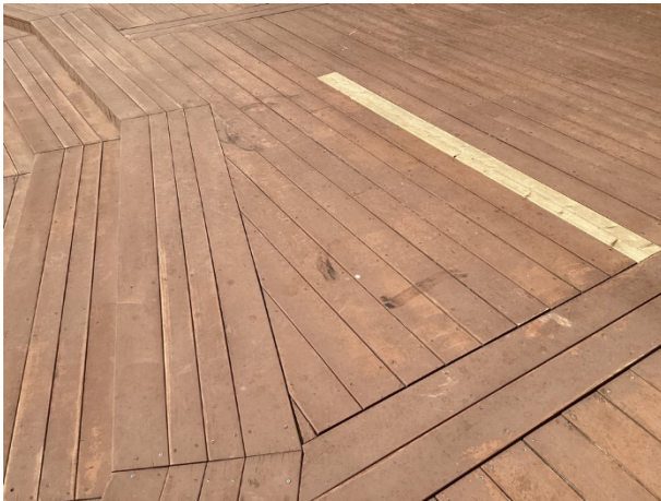
Weathered wood decking
