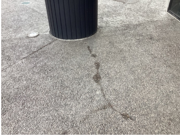
Crack at plaza
