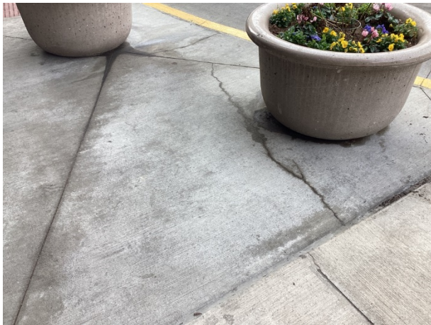
Cracks at vaulted concrete
