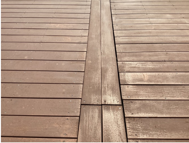
Weathered wood decking
