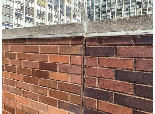
Deflection of north wall
