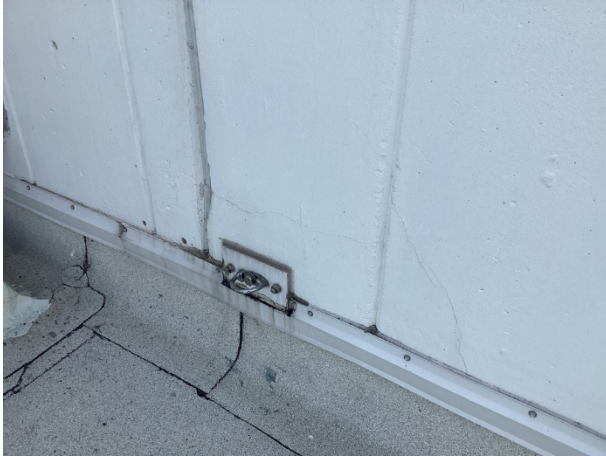
Concrete cracks at penthouse
