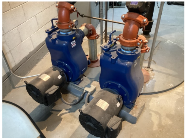
Sewage ejection pumps
