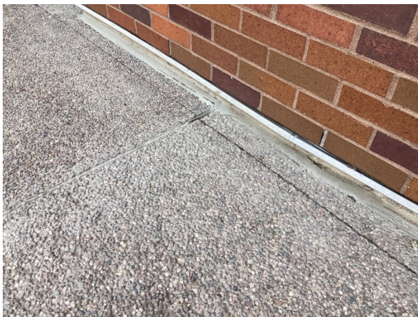
Sealant deterioration at plaza
