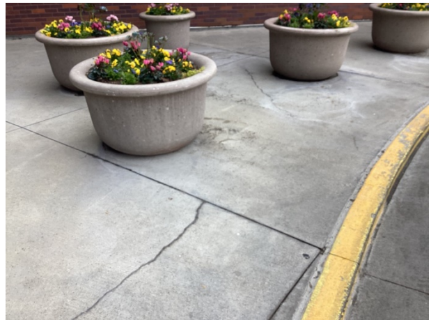
Cracks at vaulted concrete
