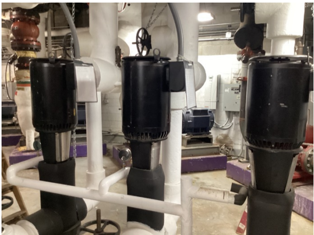
Domestic cold water pumps
