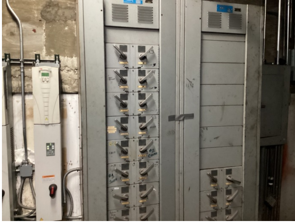
Motor control center
