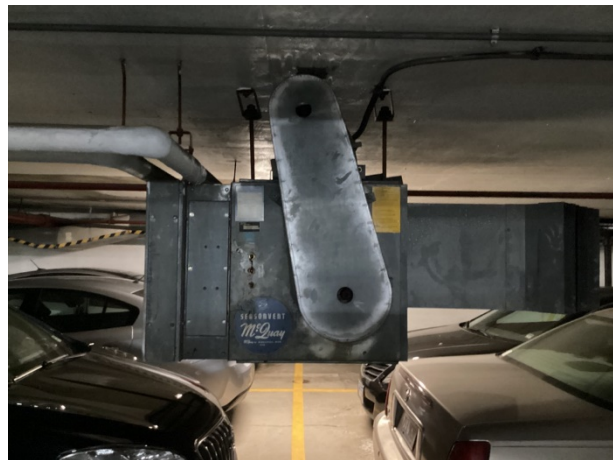
Garage air handler
