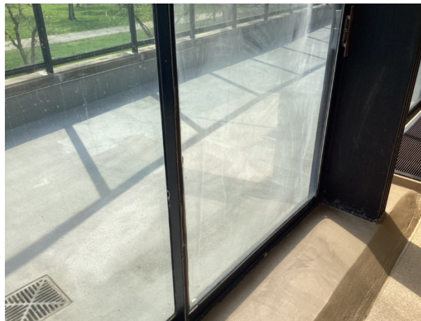
Seal failure at pool sliding door
