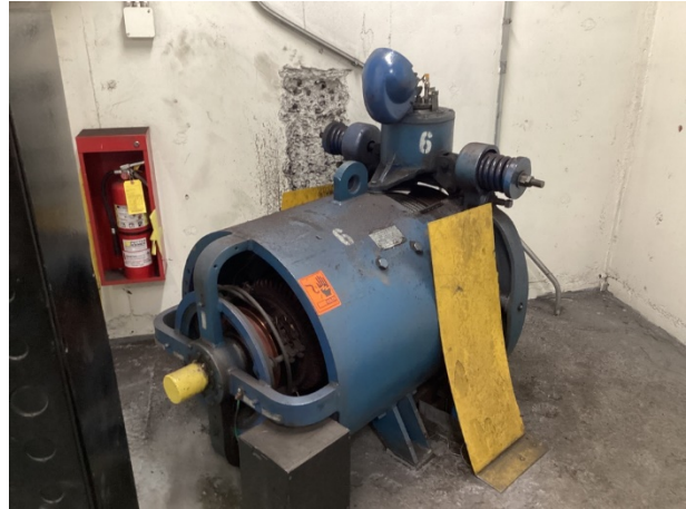
Traction elevator equipment
