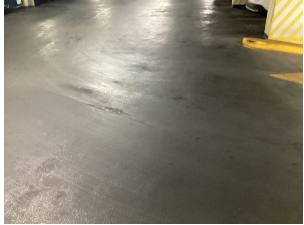
Traffic coating at turning radius
