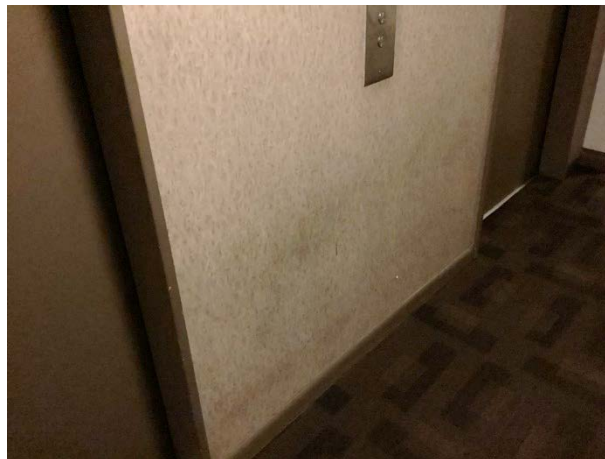
Wall covering damage
