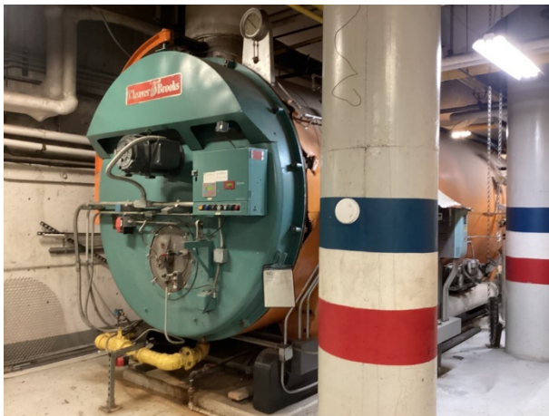
Building heat boiler
