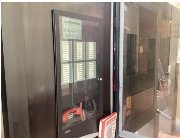
Control panels at lobby
