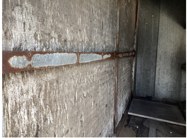
Preheat coil deterioration at hallway unit
