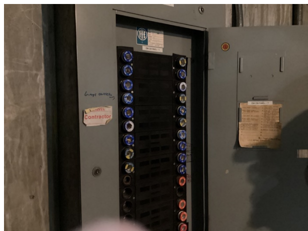
Fuse panel for garage
