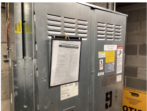
Refuse elevator controls casing
