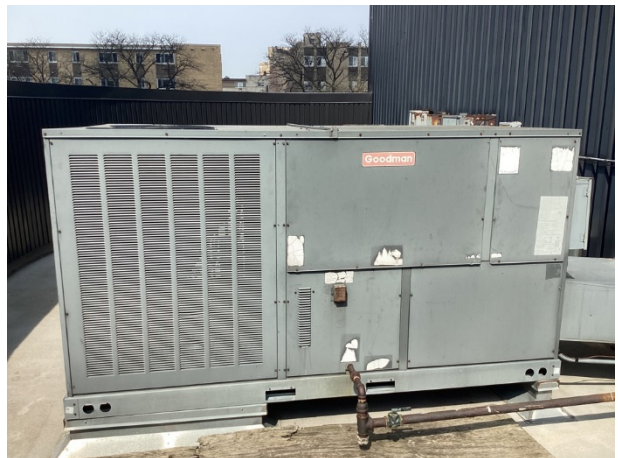
Racquetball court air handling unit
