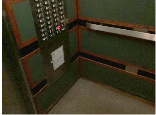
Passenger elevator cab finishes
