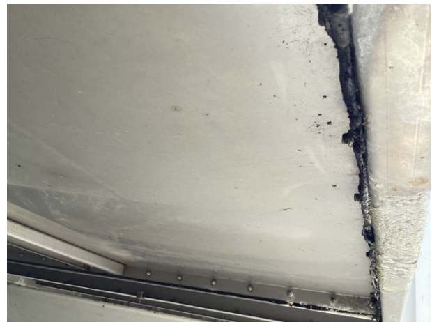
Cooling tower at leakage
