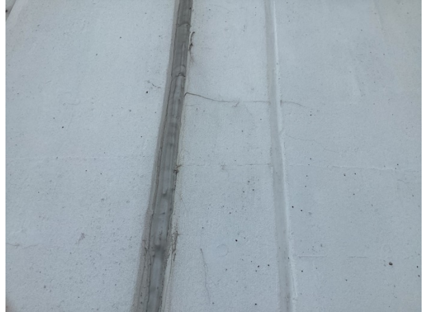
Concrete cracks at penthouse
