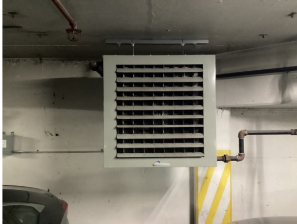
Garage unit heater
