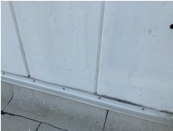
Concrete cracks at penthouse
