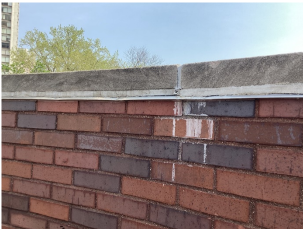
Sealant deterioration at cap
