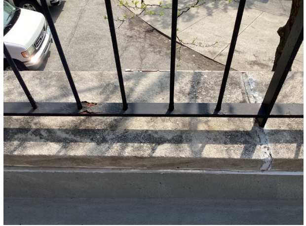
Corrosion at railing
