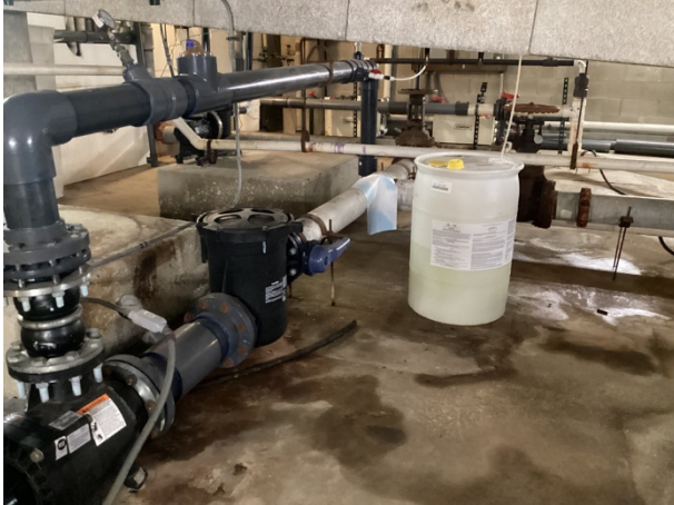
Mechanical equipment for pools
