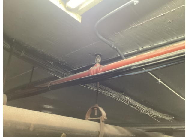
Fire suppression system
