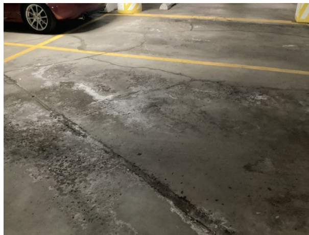
Concrete cracks and spall
