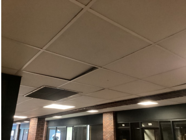
Corridor at mall ceiling tile damage
