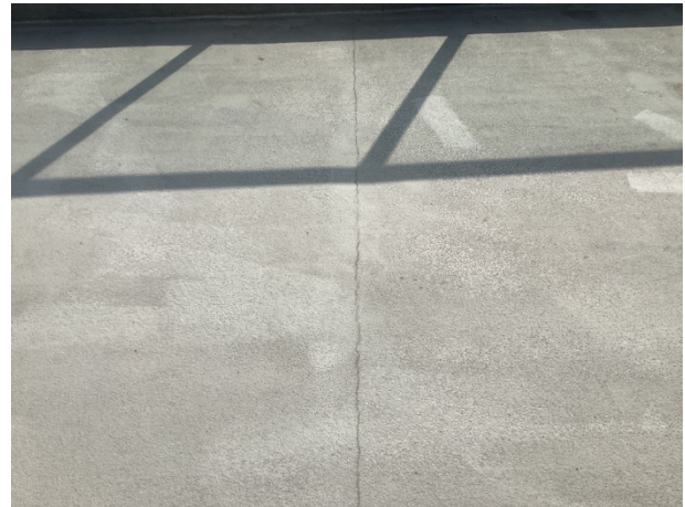
Crack at coating at 2nd floor
