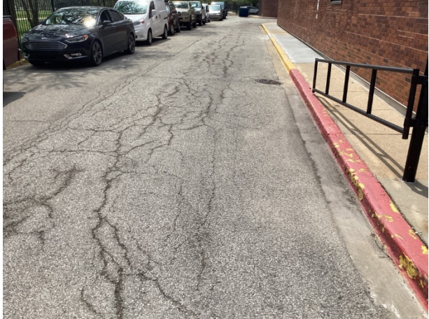
East asphalt pavement deterioration
