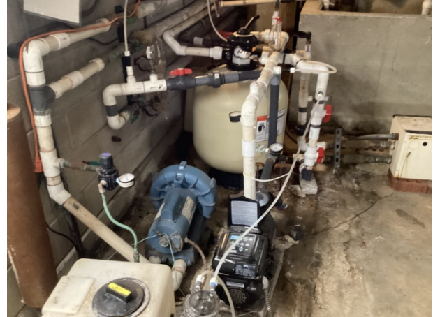
Spa mechanical equipment
