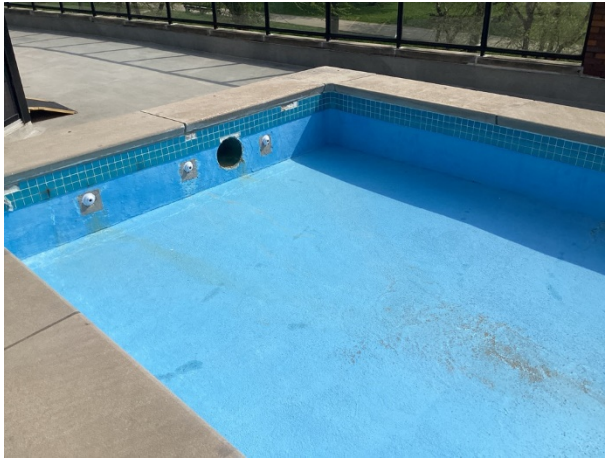
Tile damage at outdoor pool
