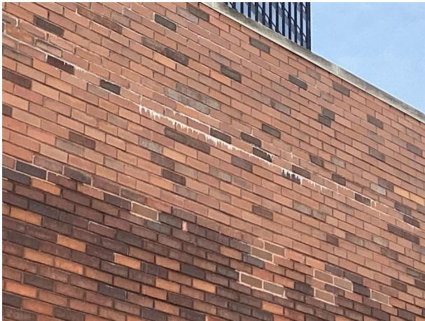
North elevation efflorescence
