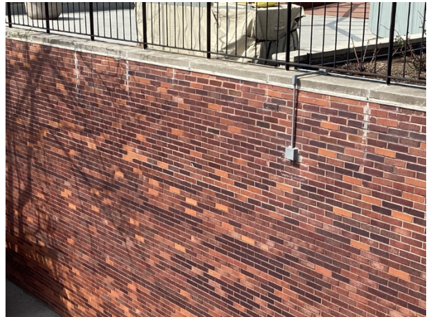
Overall deterioration of masonry wall
