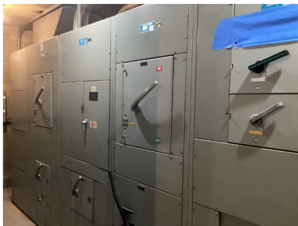
Electrical system main panels
