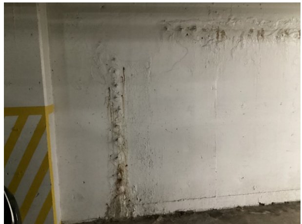
Seepage at 2P wall
