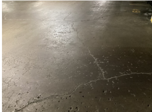
Concrete cracks and spall
