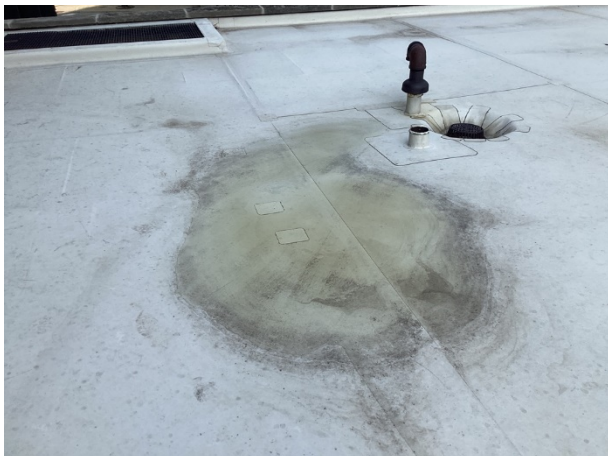
Northwest roof at 2nd floor at lack of drainage
