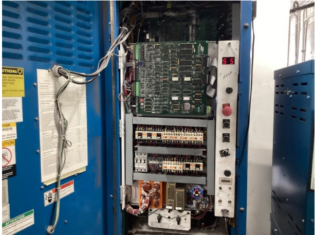
Traction elevator controls
