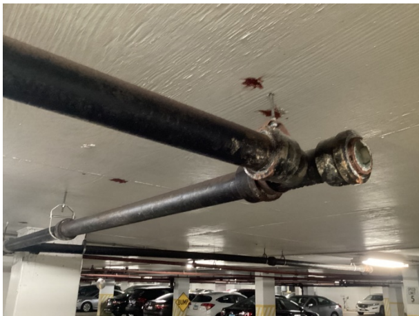
Garage drain pipe
