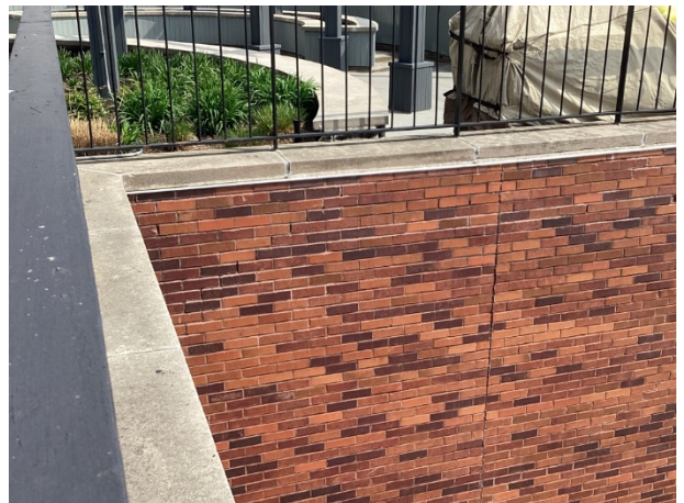
Spall and cracks at masonry wall
