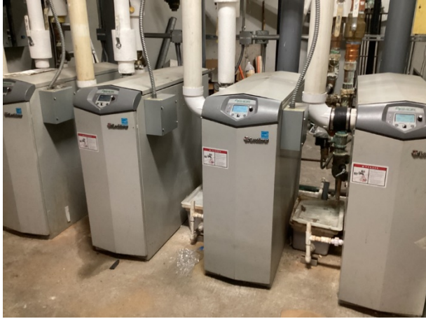
High zone domestic hot water boilers
