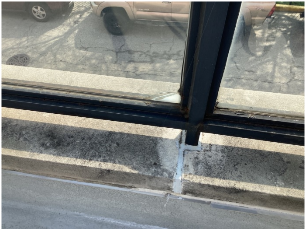
Frame corrosion and glass damage
