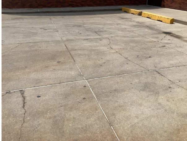
East concrete pavement cracks
