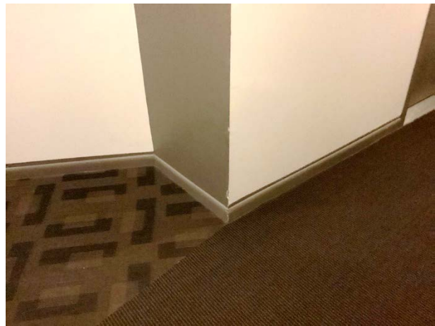
Hallway wall scuffs
