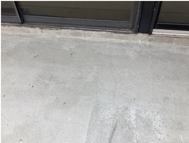
Crack at 2nd floor coating
