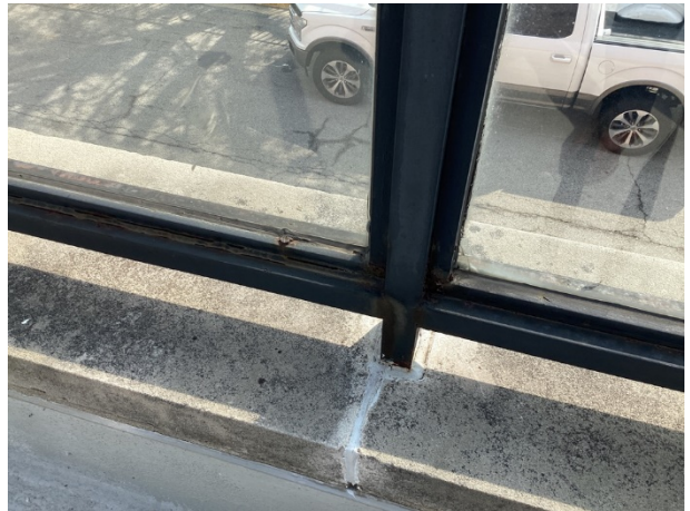
Frame corrosion and glass damage
