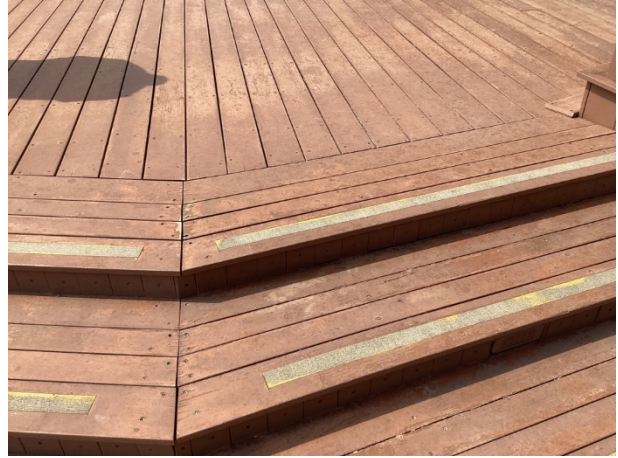
Weathered wood decking
