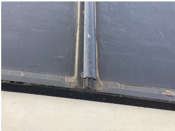
Sealants at vertical mullion
