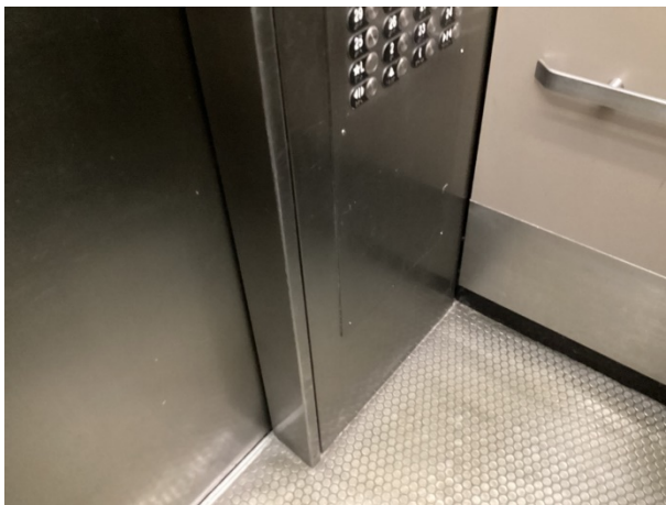
Service elevator cab
