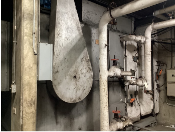
Air handling unit serving hallways
