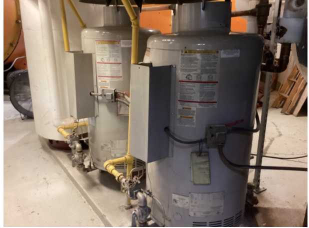
Commercial domestic water boilers
