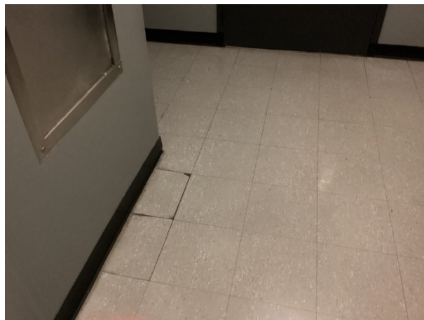
Service foyer floor damage
