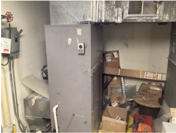
26th floor elevator room air handling unit
