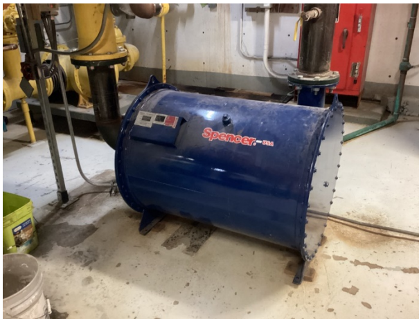
Gas booster pump
