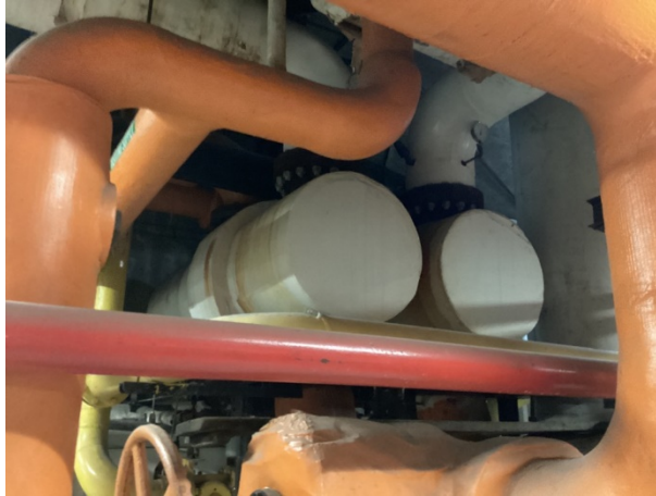
Main building heat heat exchangers
