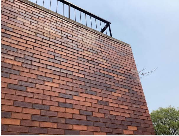
Spall and joint deterioration at masonry
