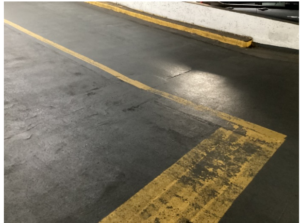
Traffic coating wear at ramp
