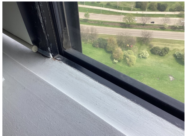
Weather strip deterioration
