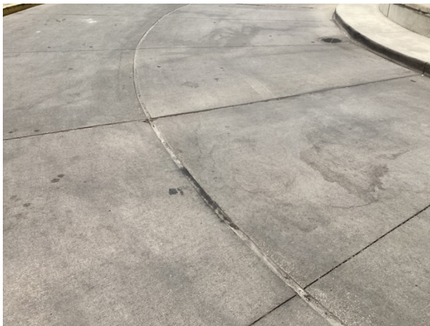
Joint sealant at pavement
