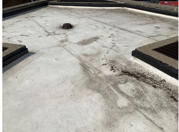
Southwest roof at 2nd floor at lack of drainage
