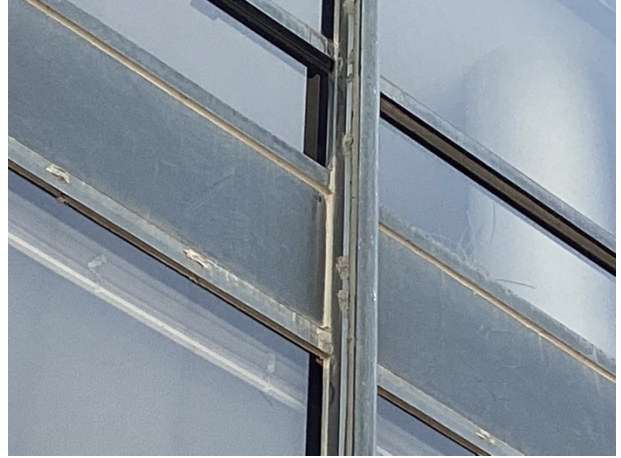
Metal to metal sealants
