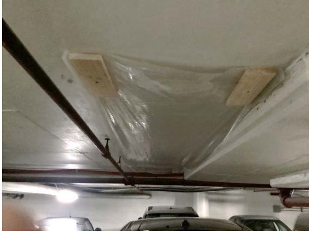
Evidence of past water infiltration beneath plaza
